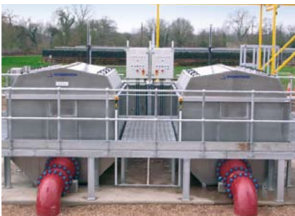
Installation at waste water treatment plant.
